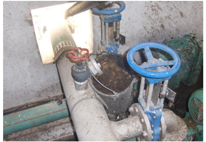
Photo 3.2: Outlet valve of sludge thickener
