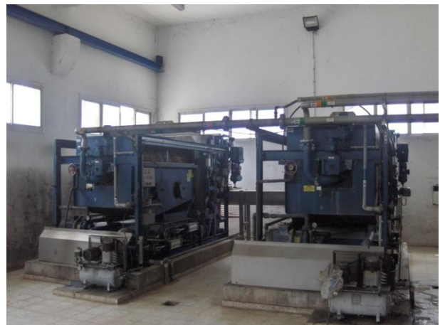
Photo 1.3: Dewatering machines at Al Bireh WWTP
